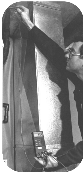
FIGURE 48 TEMPERATURE RISE MEASUREMENT
